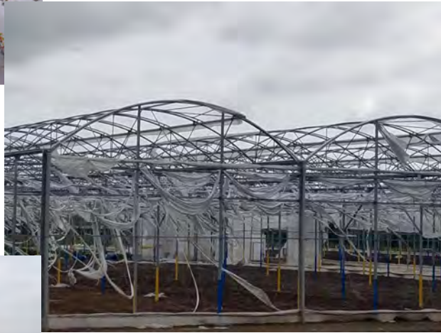
damaged infrastructure after a wind/rain event ↓
