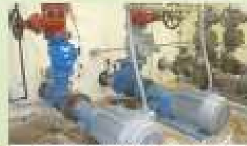
Booster Stations and Other Pumps
